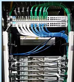
Computer room wiring
